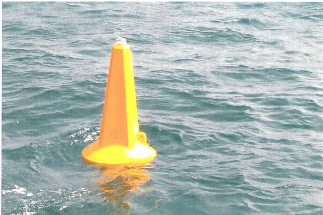
Lighted Marker Buoy installed at Marine outfall point
